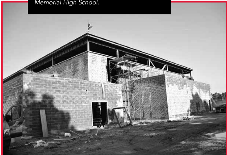
Construction progresses on the new gymnasium and locker rooms at Amityville Memorial High School.
